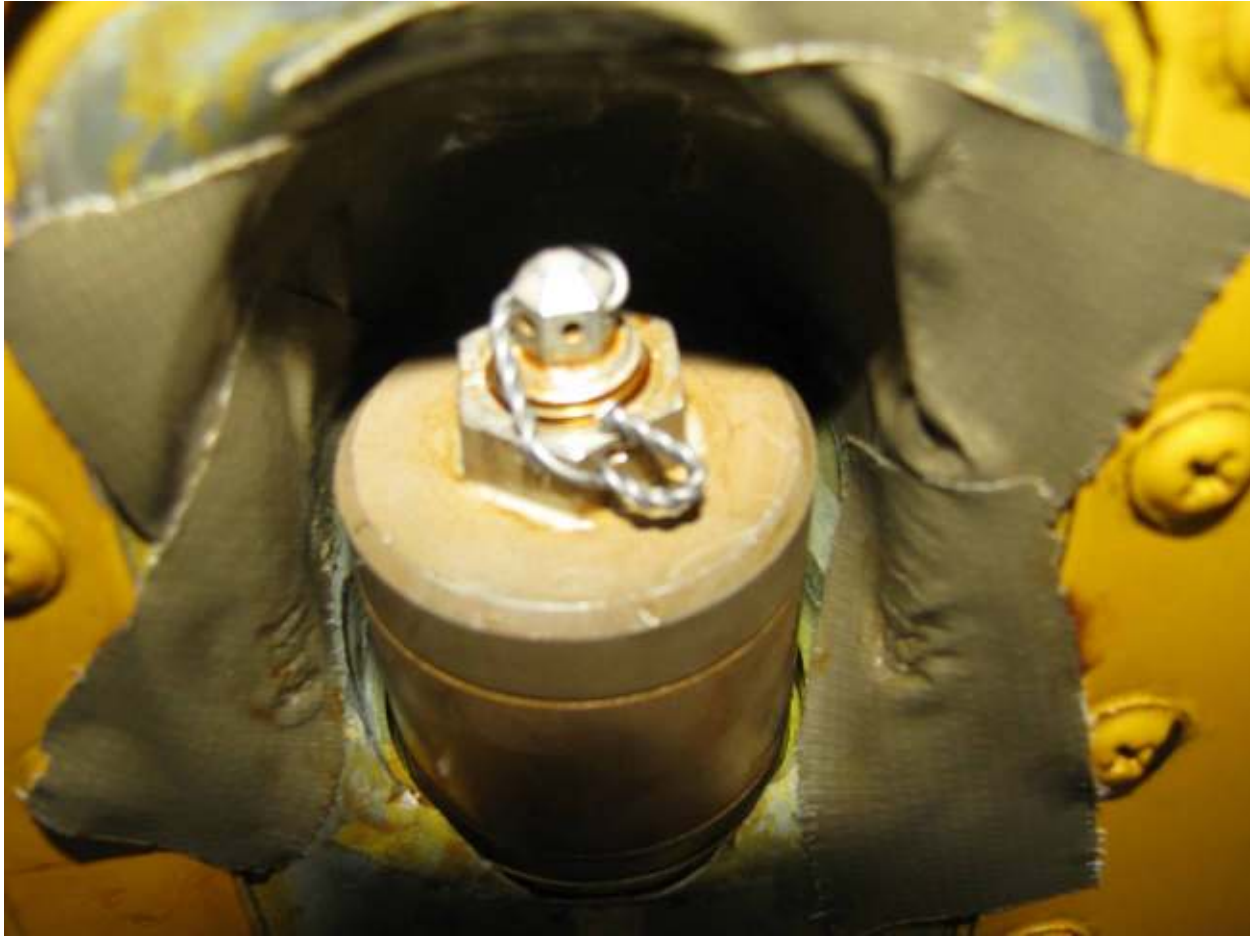
Fig. 11. Properly installed and torqued ALEC cable. Each side is symmetrical at the bath tub fitting and internally with respect to the thread engagement into the swage fitting. The tension nut, above, has been rotated 4½ turns after a pre-torque of 50 in-lbs has been applied to the tension nut.
